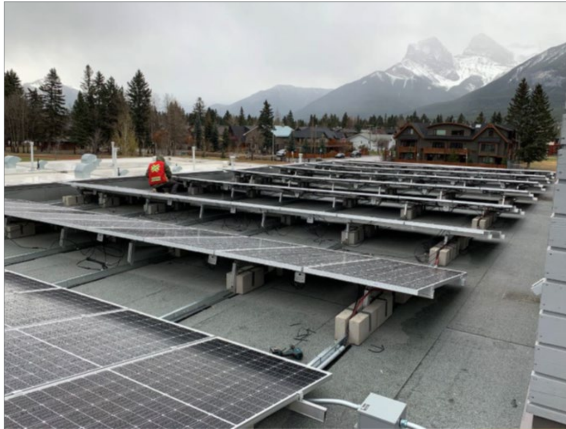
Ballasted solar PV array at Lawrence Grassi Middle School.
