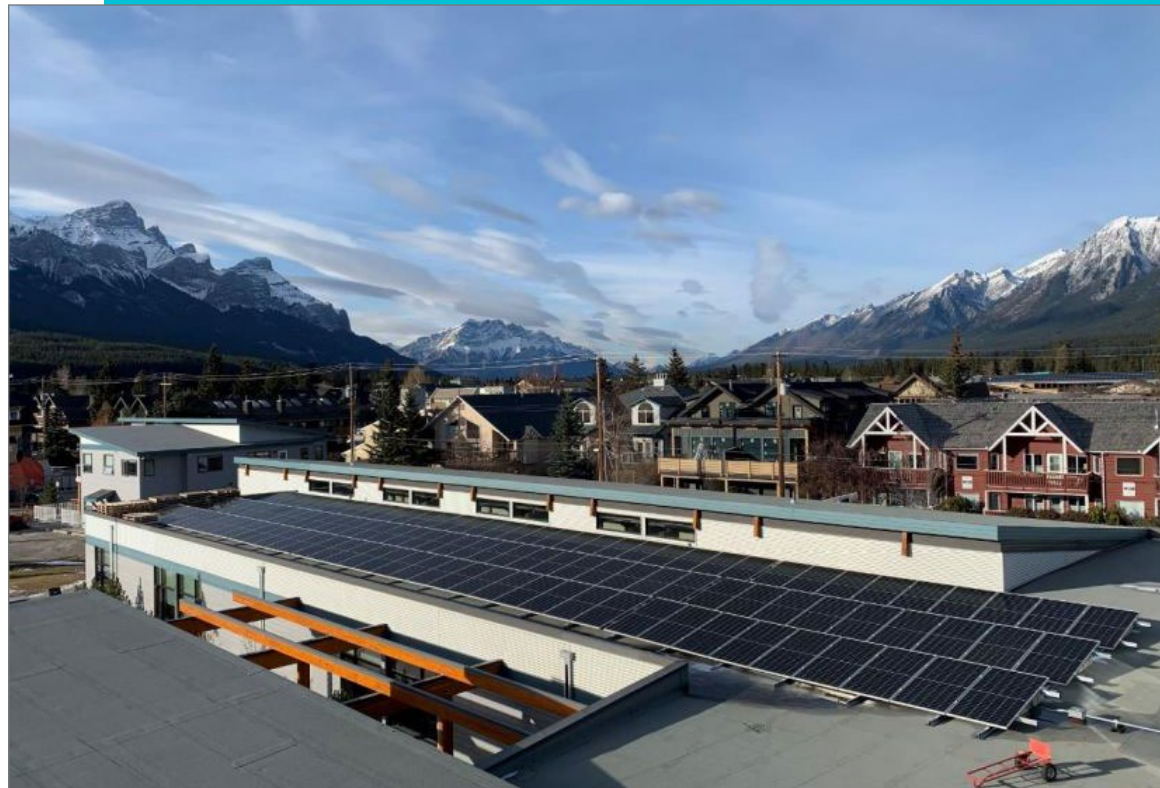
A portion of the solar PV array at Lawrence Grassi Middle School.
