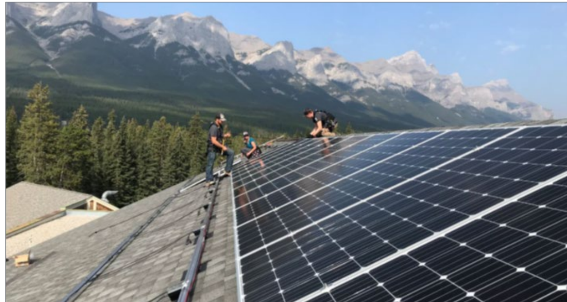
Installers working on the solar PV array at Canmore Collegiate High School.
