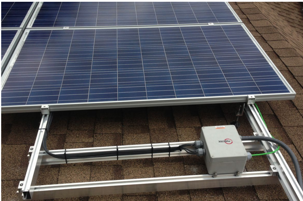
Figure 7: Solar PV system cabling and combiner box Photo: Green Sun Rising
