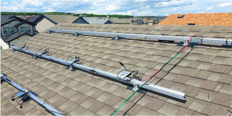
Figure 14: Solar PV racking on sloped asphalt roof Photo: SkyFire Energy
