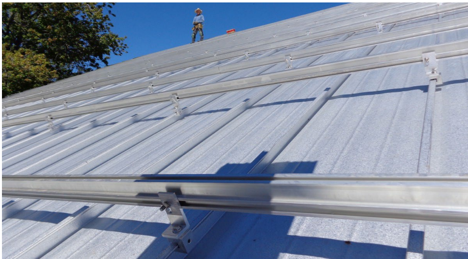
Figure 15: Solar PV racking on lightweight metal roof Photo: Green Sun Rising
