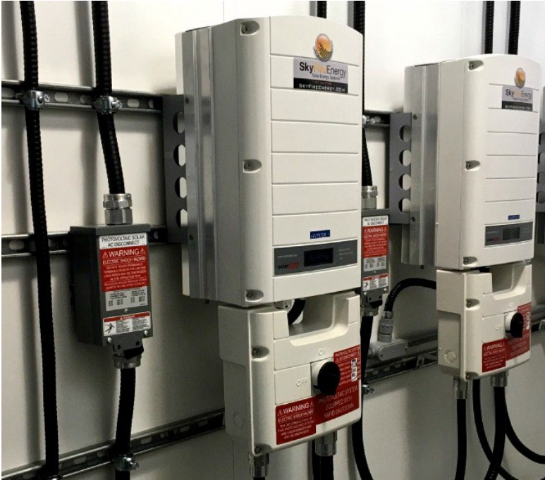
Figure 8: Solar PV system disconnects and electrical panels Photo: SkyFire Energy.
