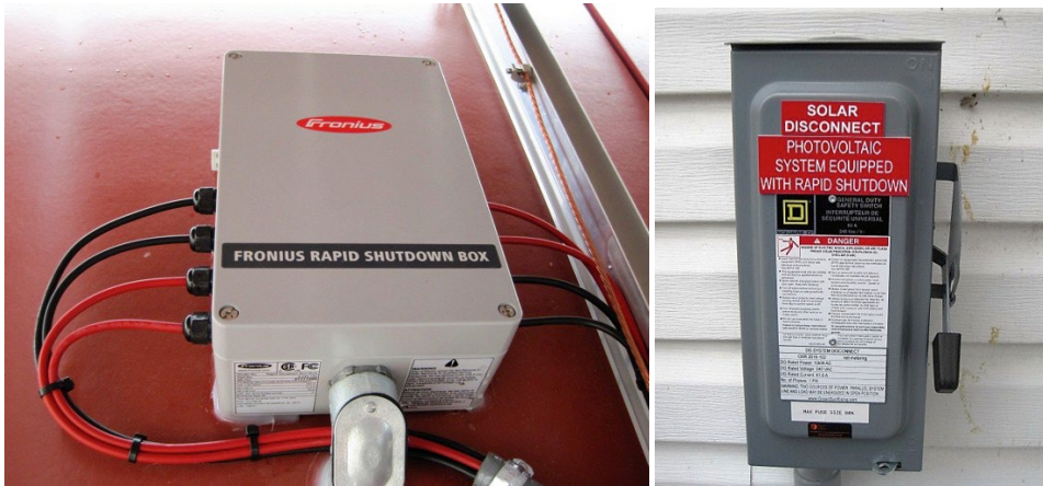
Figure 9: Rapid shutdown device (left) and DC disconnect with appropriate labeling (right) Photo: SkyFire Energy and Green Sun Rising
